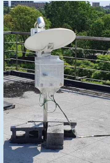
Microwave Rainfall Radar
